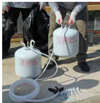
Shaking of A-side and B-side tanks
